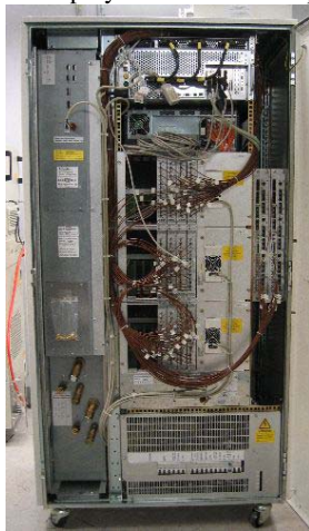
Figure 1: Additional electronics cabinet for seamless integration of additional 96 receivers
