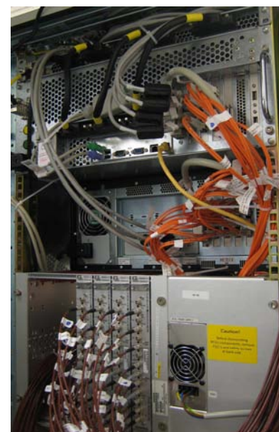
Figure 2: Picture of the top half of the extension cabinet showing the MRIR, PCI Extender box and one of the additional chassis with 4 receiver boards
